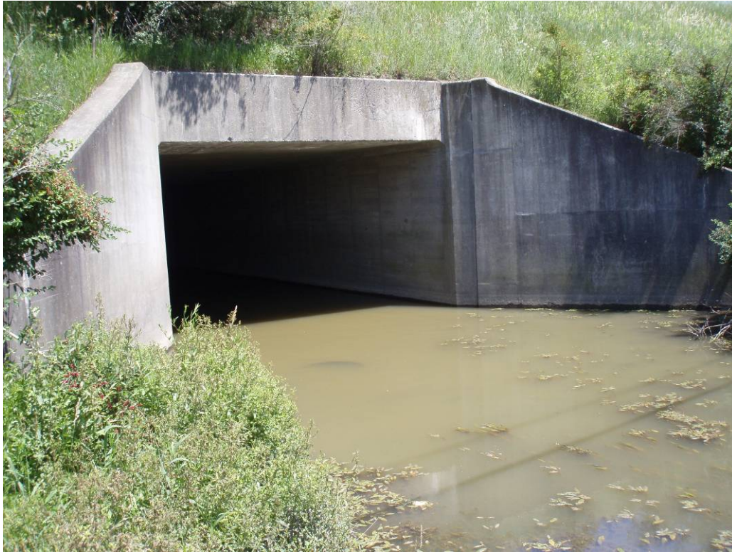
PHOTO 5. Reach 2, Carpenter Creek downstream concrete box culvert at Route 17M, view to east.
